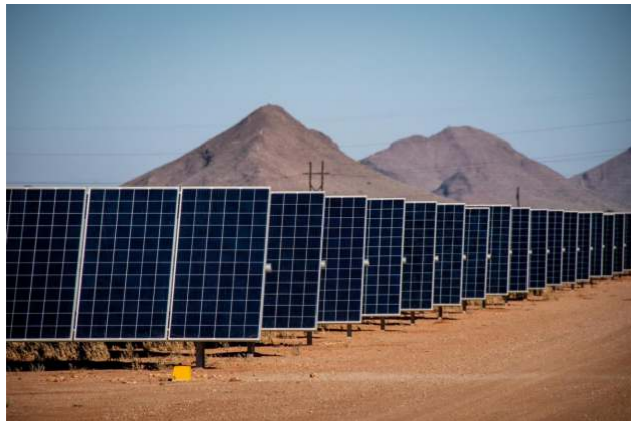
South Africa: Two large-scale solar plants begin feeding green power to the national grid.
