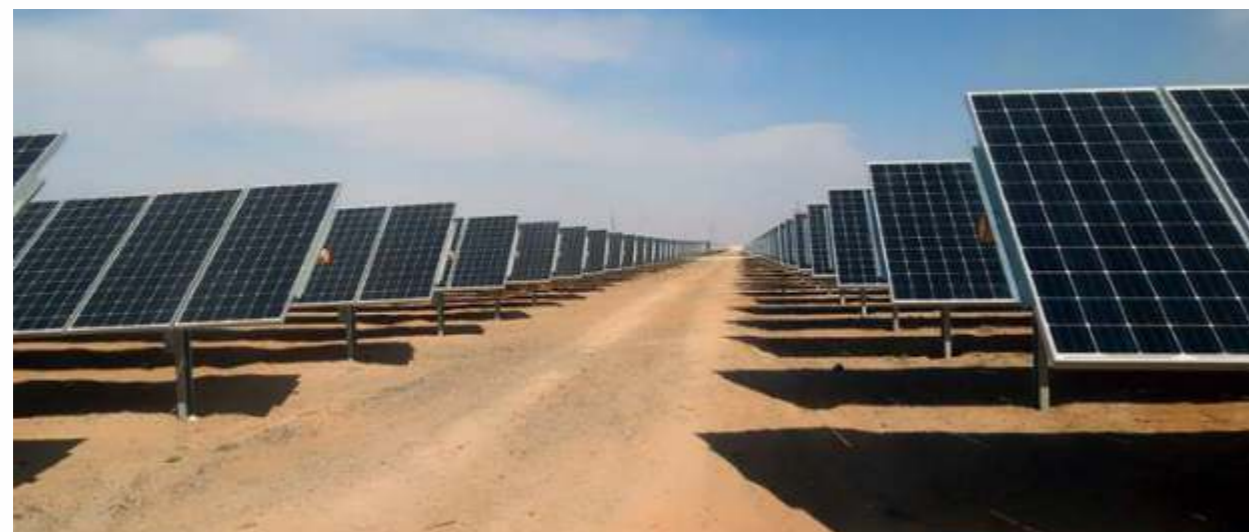
A solar power plant.
