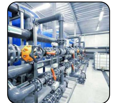
Plumbing, Sewer, & Drainage Systems
