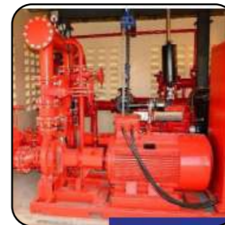
Fire pump sets and hydrant systems
