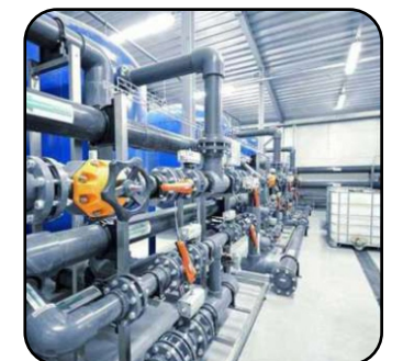
Plumbing, Sewer, & Drainage Systems
