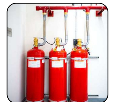
Automatic Fire Suppression Systems
