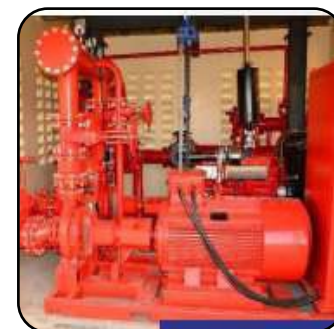
Fire pump sets and hydrant systems
